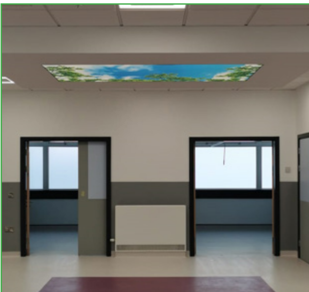
Atkore Marco Name: Craigavon Area Hospital Vertical Market: Health Care Products Used: Marco Elite 3 Hygieia
