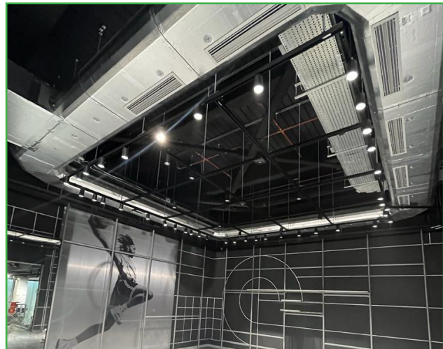
Atkore Unistrut Name: Ahead of the curve Vertical Market: Retail Products Used: P1000T and fixing accessories
