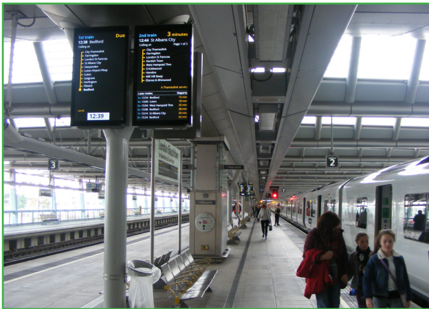
Atkore Flexicon Name: Thameslink Vertical Market: Rail Products Used: LFHUBRD Conduit System
