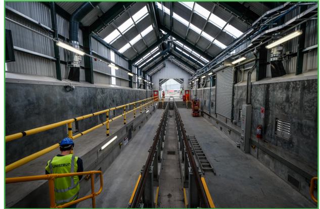
Atkore Unistrut & Flexicon (APAC) Name: Kiwi Rail Vertical Market: Rail Products Used: Cable Ladder
